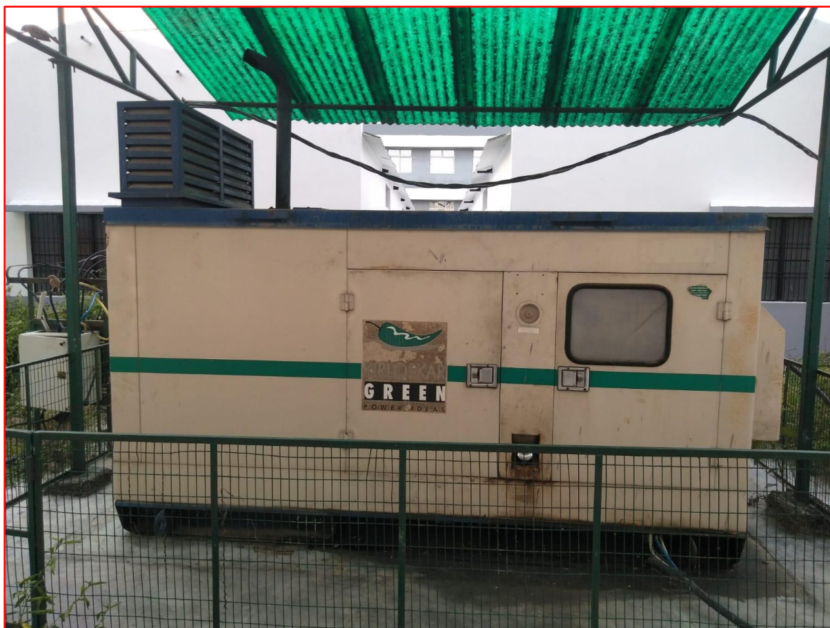
Photograph of D.G. Set installed in Campus Area
